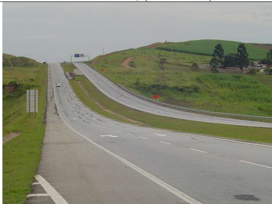
Foto 68 – Asfalto irregular – km 118,0
